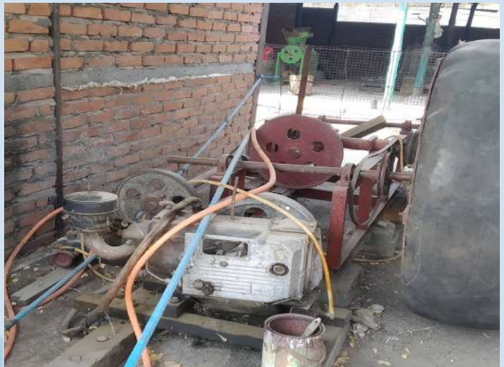
An Old Diesel Generator
